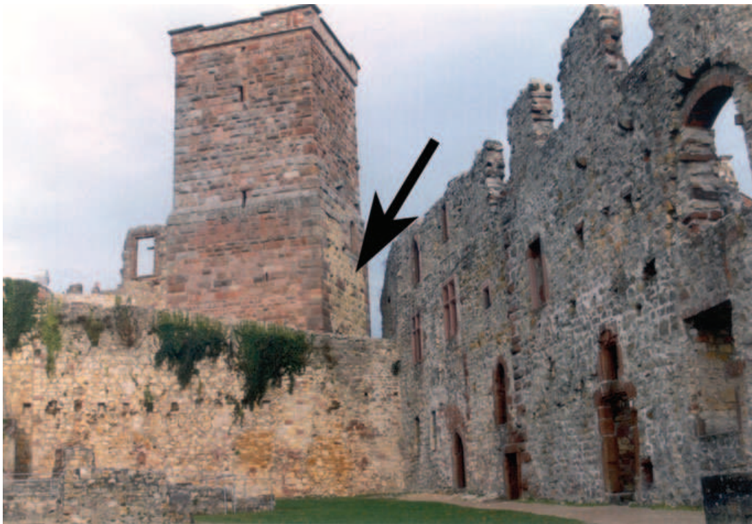
Figure 9. Picture of Rötteln Castle close to Lörrach (Schomann, unpublished data). See noticeable repairs on its eastern side (see arrow). Documents providing reasons for the repair do not exist.
