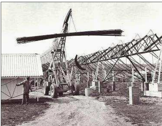
Figure 4: Erection of the East arm reaches the centre. The insulated phasing hut is on the left.
